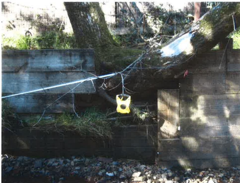
Photo 1. View to near downstream end of existing left bank retaining wall replacement project limits approximately 65 feet downstream from Norwood Avenue Bridge (January 2015). Note partially failed condition of wall segment immediately upstream from the forked maple tree to be removed by the project.
