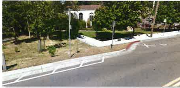
2 Westbound sidewalk gap on Lagunitas Rd.
