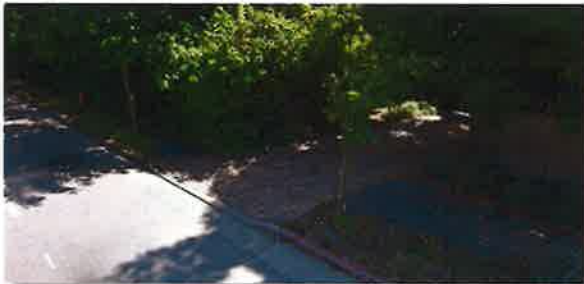
4 Southbound sidewalk gap on Poplar Ave.
