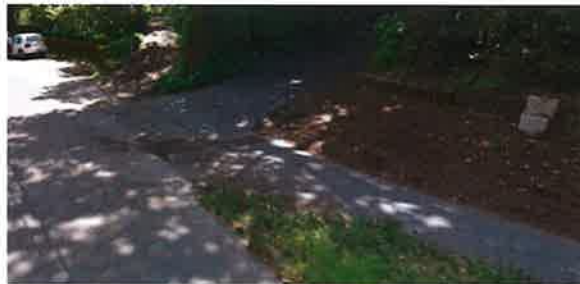
5 Eastbound sidewalk gap on Lagunitas Rd.
