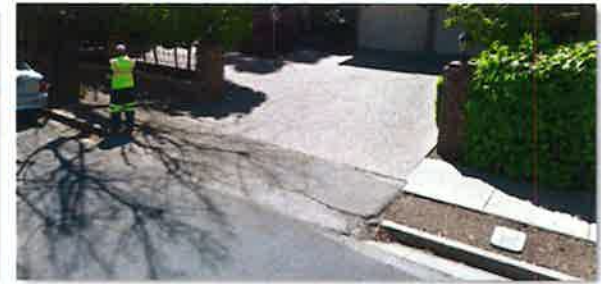
3 Southbound sidewalk gap on Redwood Dr.
