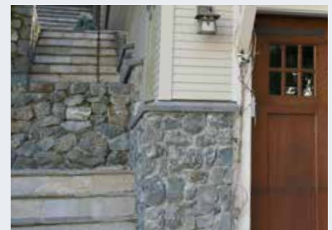
Masonry, such as stone or brick
