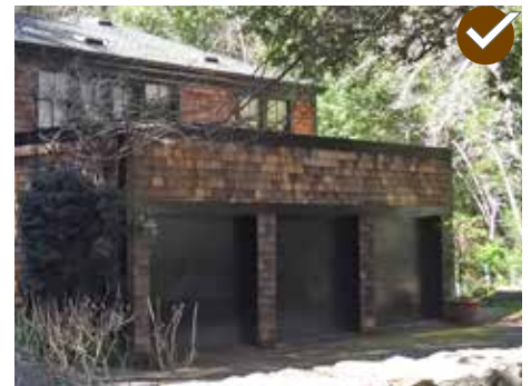
When feasible, use separate, single-car entrance doors rather than a single two-car or (three-car) entrance door.
