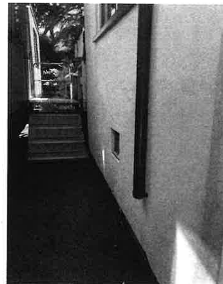
Unconnected rain water leader.
