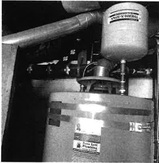
Fire House Water Heater
