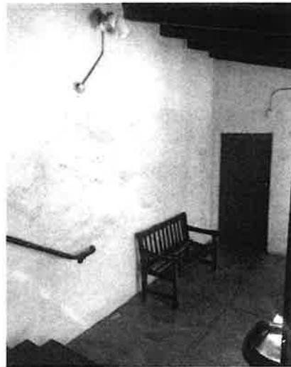
Faded plaster paint
