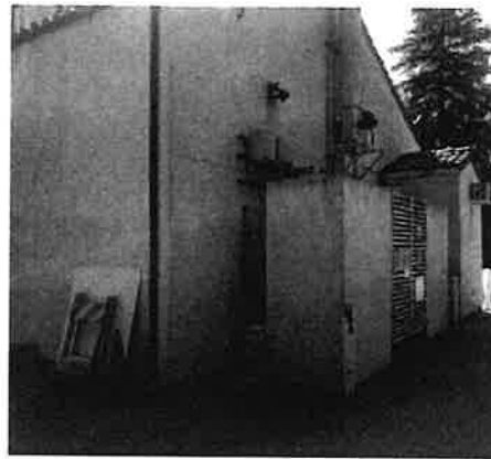
Cell tower equipment
