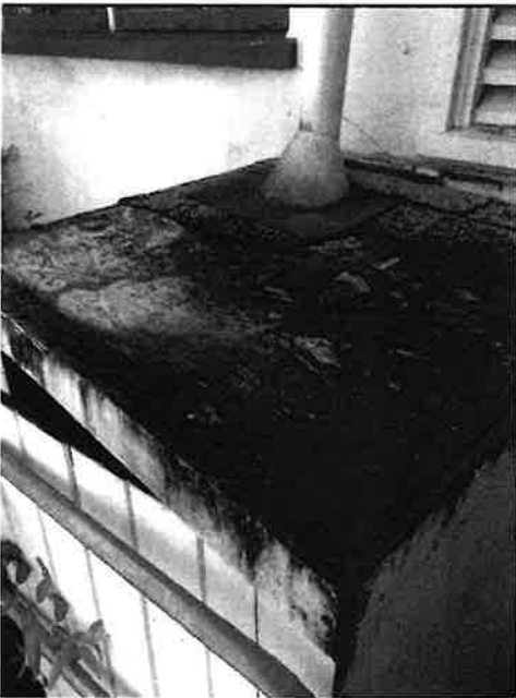
Roofing needs replacement
