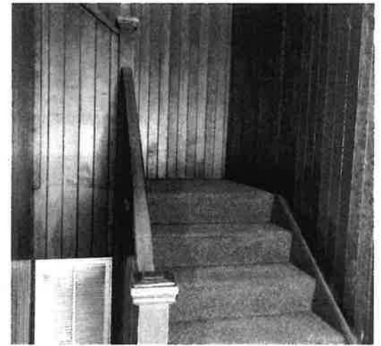
Non-compliant ADA stairs
