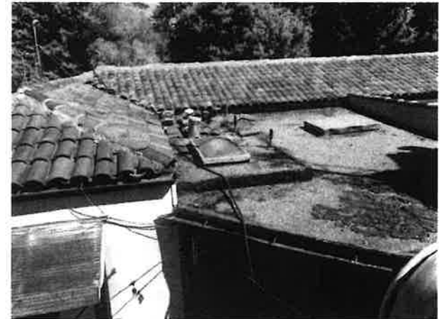
Roofing in need of repair, misc. exposed wiring.
