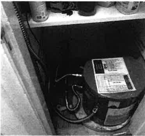
Police Station Water Heater
