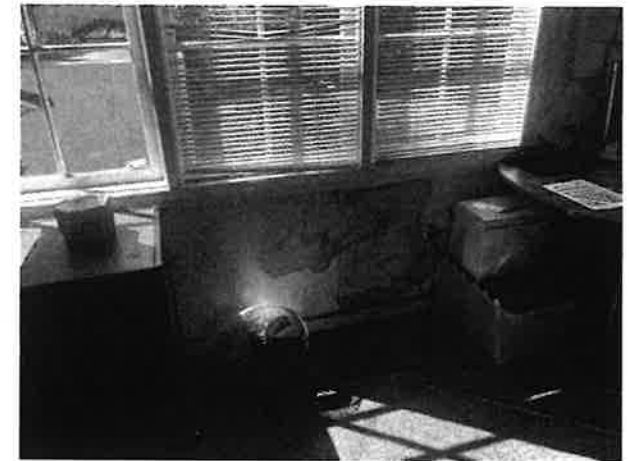
Water damage at exterior wall
