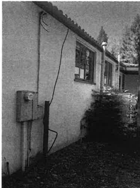
Soil contact with plaster
