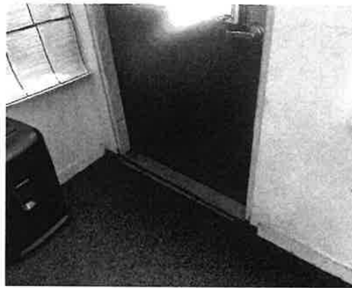
Water staining at threshold
