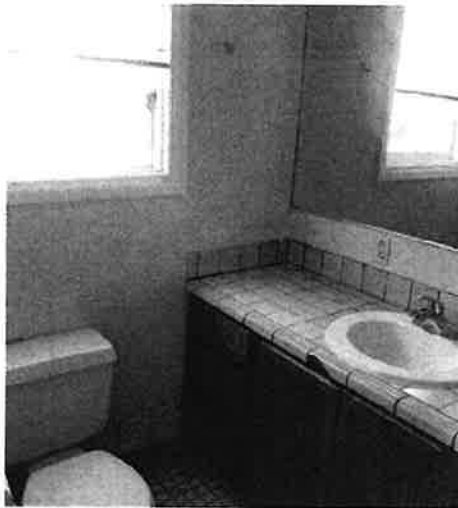
Broken counter top tile
